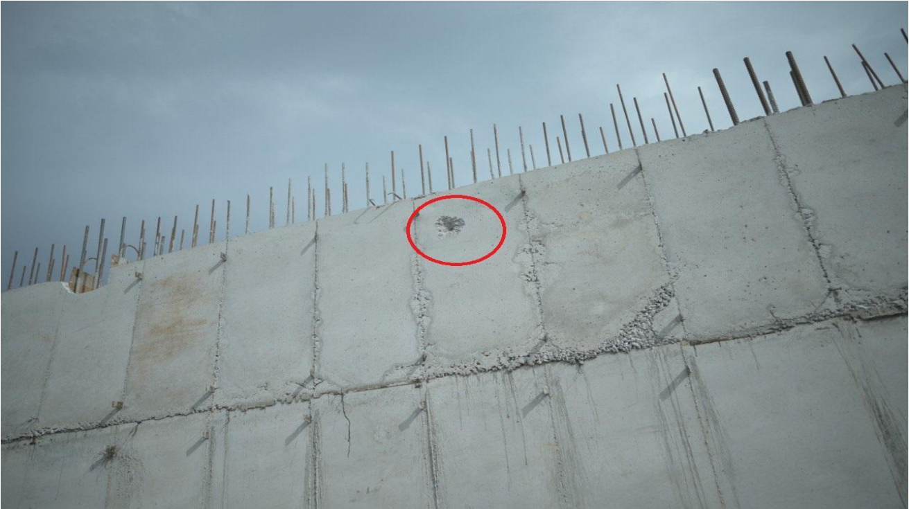
Photo 8.1: Damage to the newly built walls, columns and fence of the Plant
